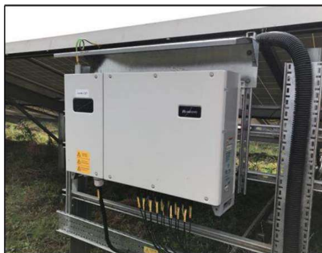
Figure 2-1: Typical String Inverter
