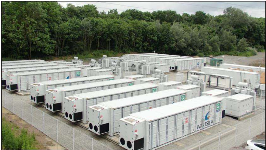
Figure 2-4: Example BESS facility
